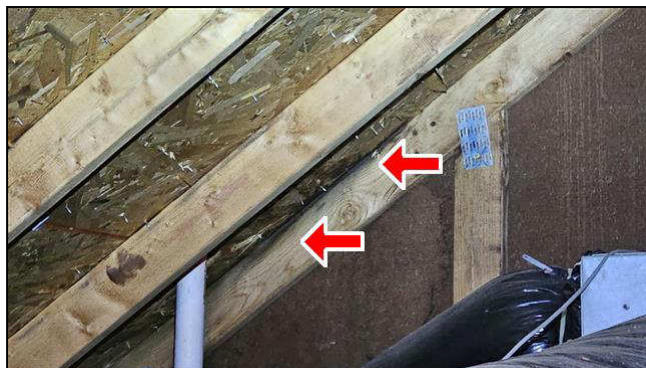
F. Item 3(Picture) rear right roof
