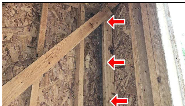
D. Item 1(Picture) rear right corner of crawlspace
