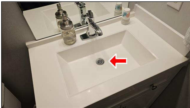
A. Item 5(Picture) upstairs hall bathroom sink
