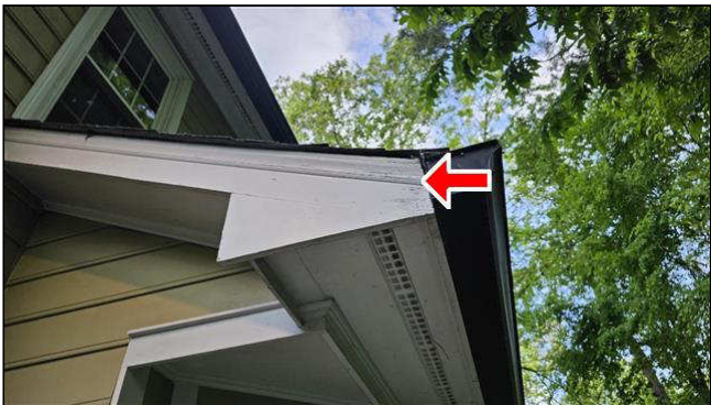
F. Item 4(Picture) rear shed roof
