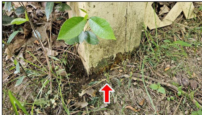
D. Item 1(Picture) rear deck
