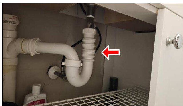
A. Item 2(Picture) upstairs hall bathroom sink
