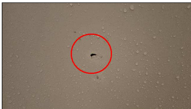
B. Item 2(Picture) upstairs hall bathroom tub
