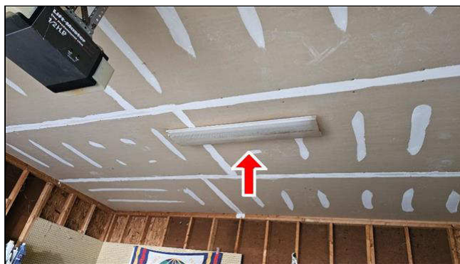
D. Item 1(Picture) garage
