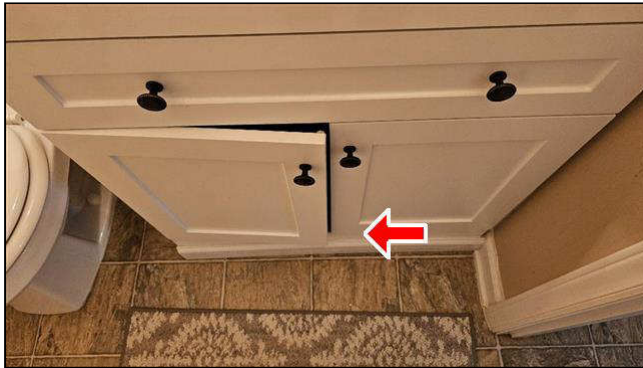
E. Item 1(Picture) downstairs bathroom sink
