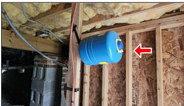
C. Item 1(Picture) water heater in crawlspace
