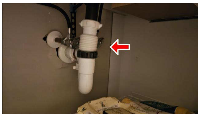
A. Item 1(Picture) downstairs bathroom sink
