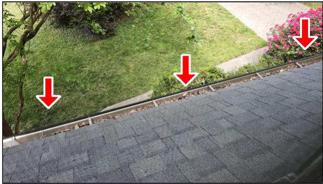
D. Item 3(Picture) front porch roof
