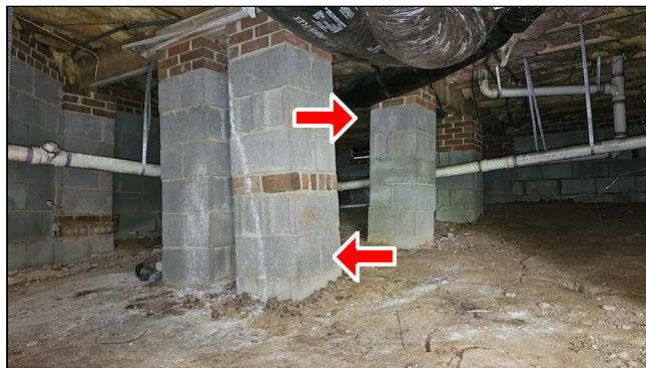
C. Item 1(Picture) under front entry
