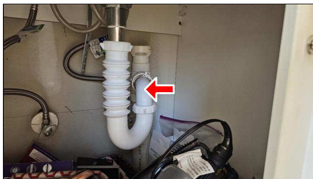
A. Item 3(Picture) primary bathroom right sink
