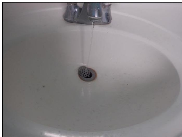
Drain stop missing/ineffective
