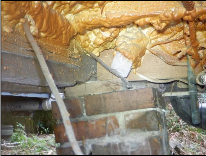
Excessive, or improper shims
