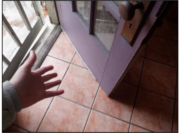
General door issues
