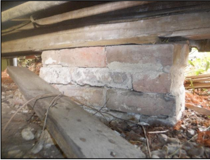
Mortar and/or brick deterioration
