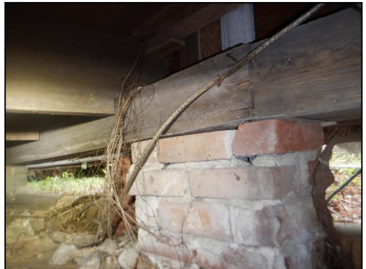
Mortar and/or brick deterioration
