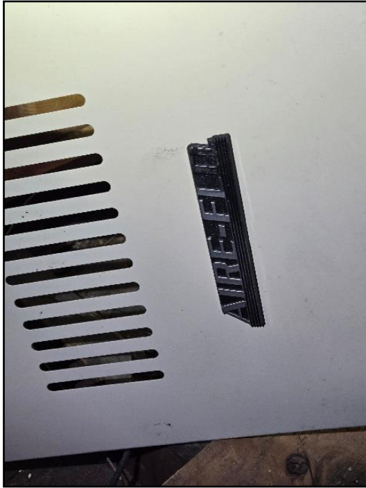
General View of Heating System
