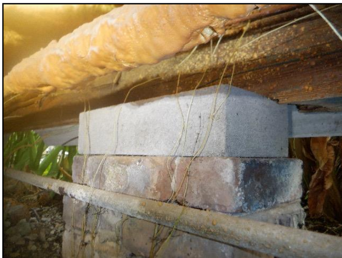
Excessive, or improper shims
