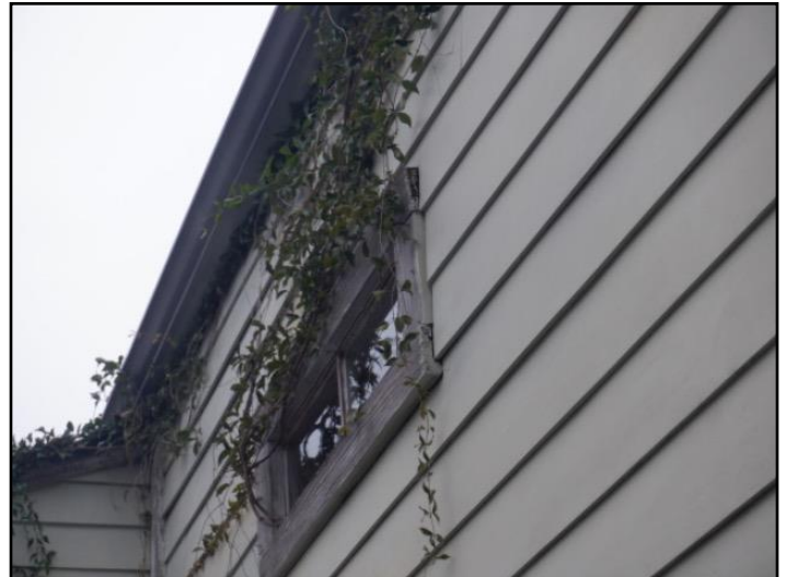
Vines can damage siding by trapping moistur...
