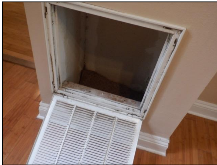
Filter missing, wrong size or collapsed
