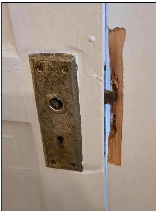
General door issues
