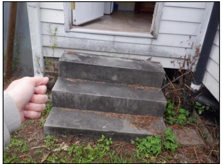
Missing stair handrail
