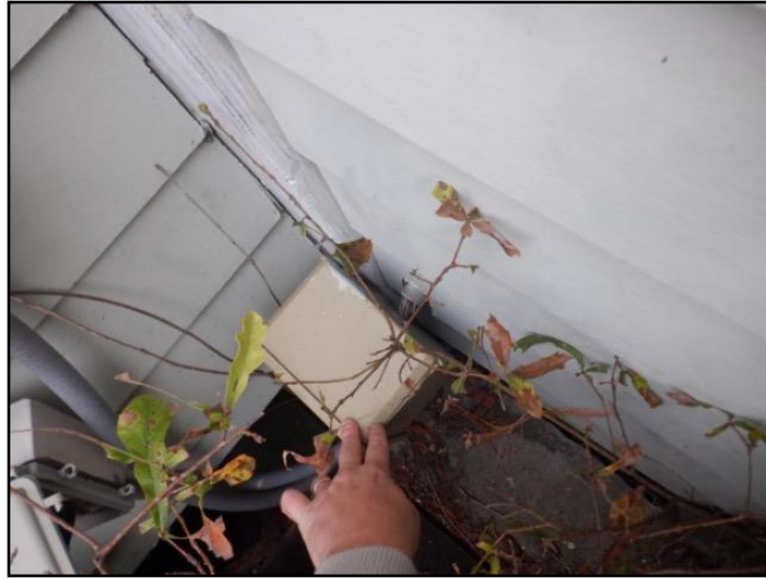
Loose conduit, exposed wire
