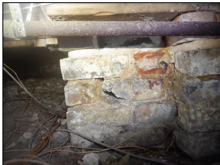
Mortar and/or brick deterioration
