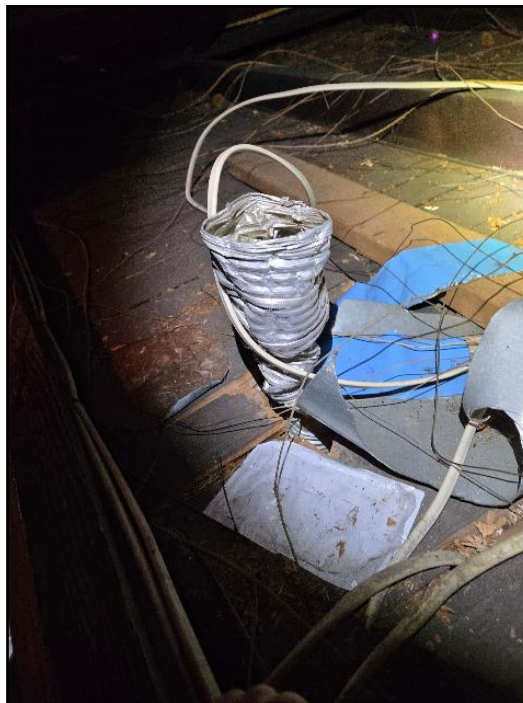
Not vented to exterior
