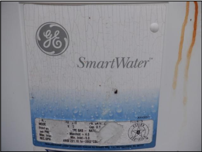
General View of Plumbing System
