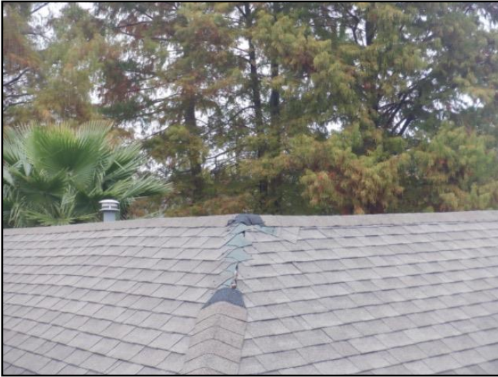
Missing, loose or torn
