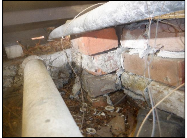
Loose or missing brick or block
