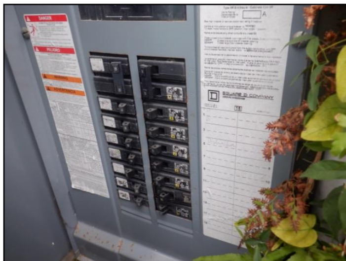
Circuits not labeled
