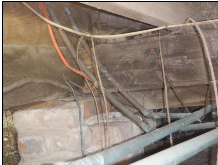
Loose or missing brick or block
