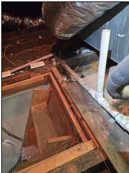
Line not insulated
