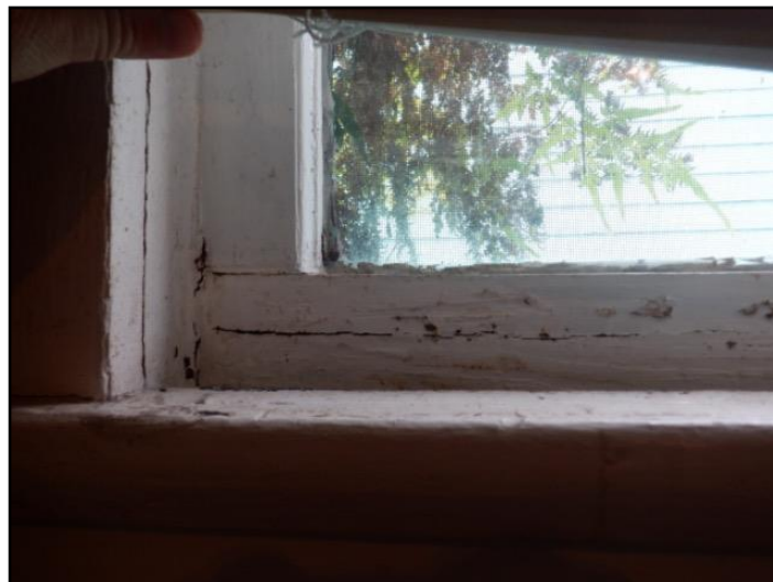
General window issues
