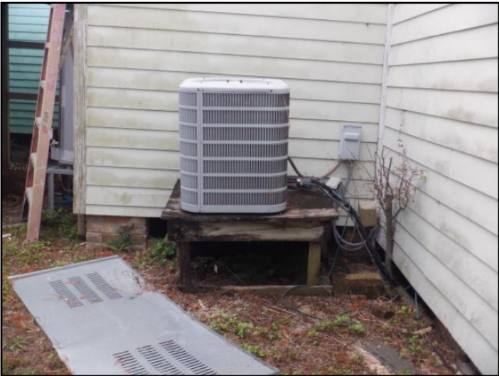
General View of the Cooling System
