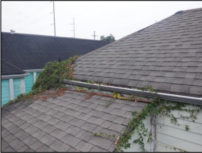
Vines on roof covering
