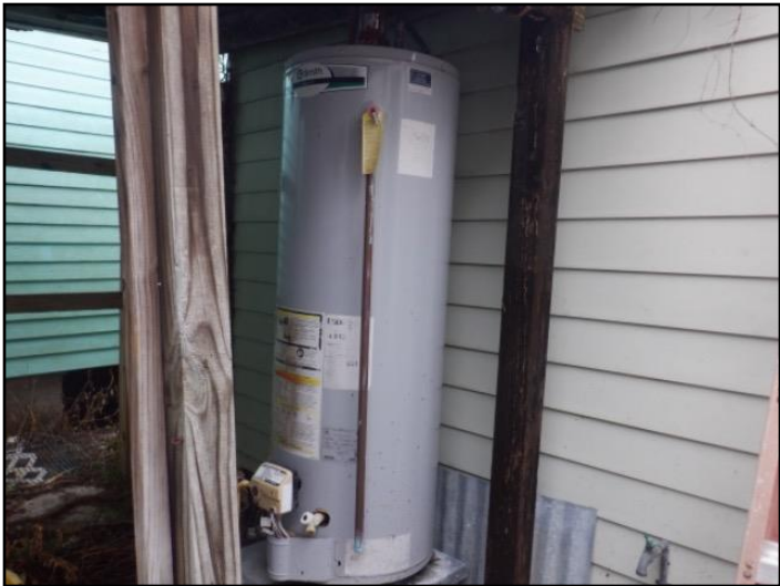
General View of Plumbing System
