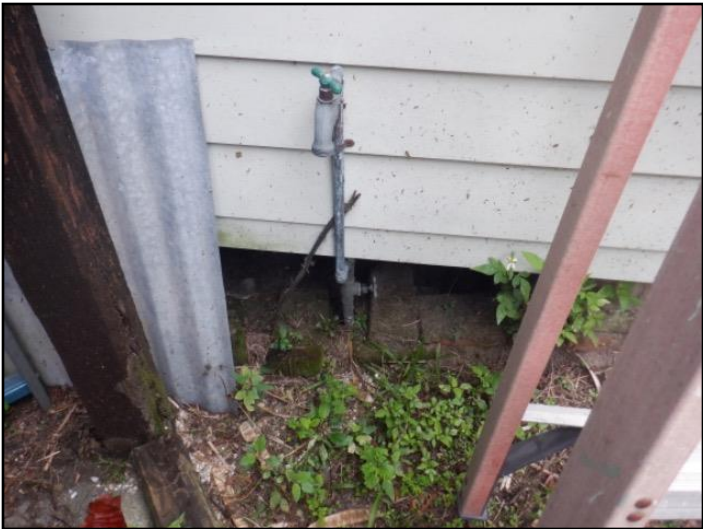
General View of Plumbing System
