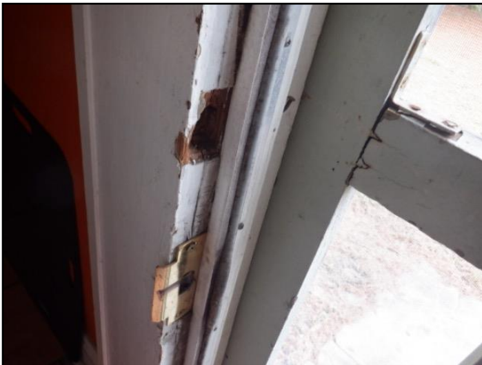
General door issues
