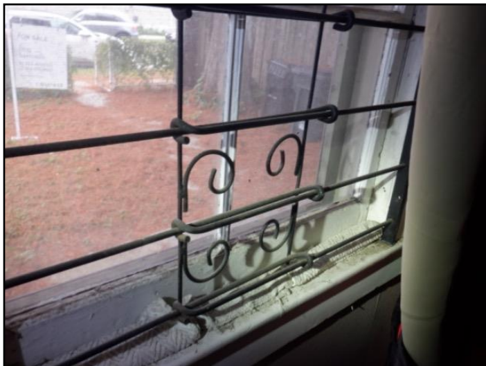
General window issues
