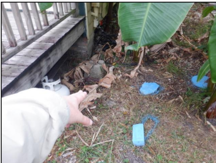
Improper slope or drainage
