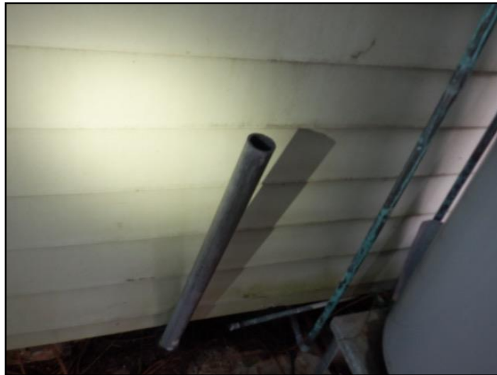
The vent terminates too low
