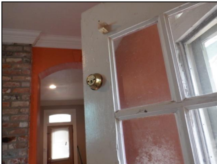
General door issues
