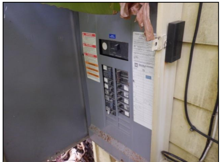
General View of the Electrical System
