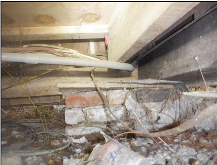
Excessive, or improper shims
