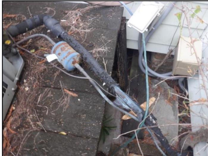
Old and/or damaged insulation
