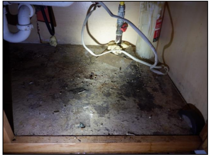
General cabinets and countertop issues
