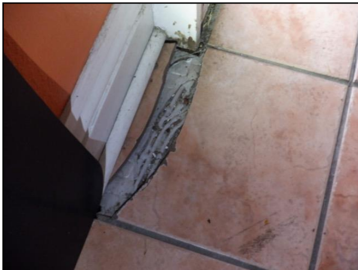
Tiles/grout loose cracked, broken, or missing
