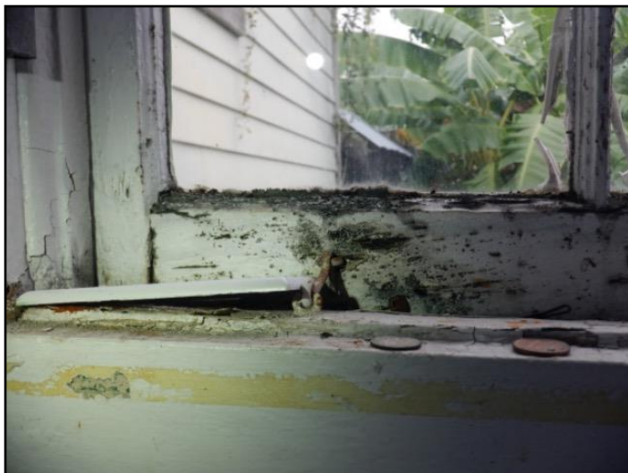
General window issues
