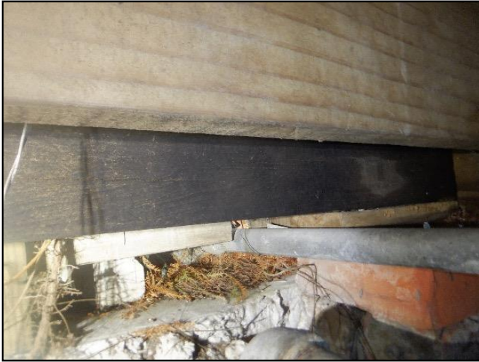
Excessive, or improper shims
