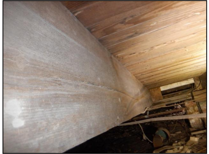
Split or damaged
