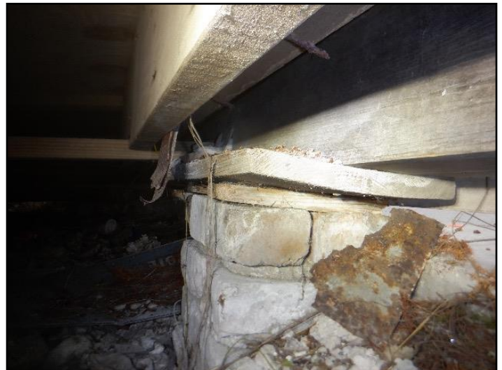
Excessive, or improper shims
