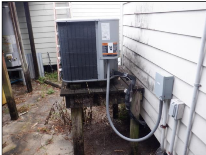
General View of the Cooling System
