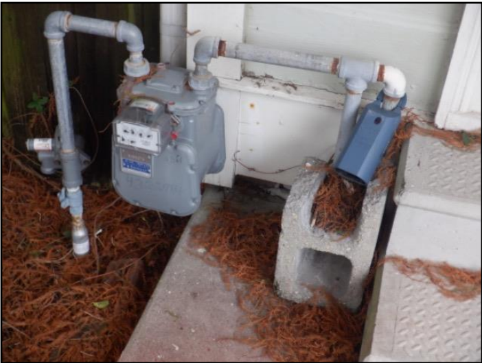
General View of Plumbing System
