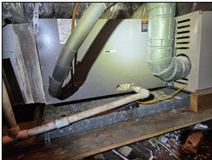
General View of the Cooling System
