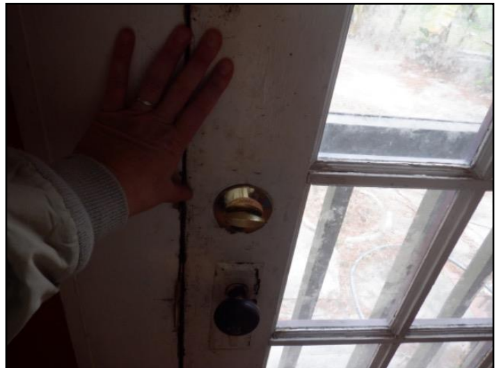
General door issues
