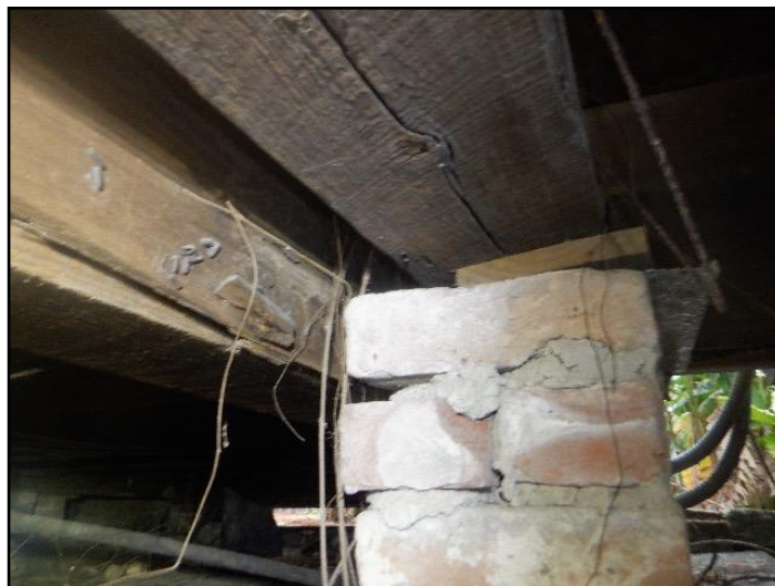
Excessive, or improper shims
