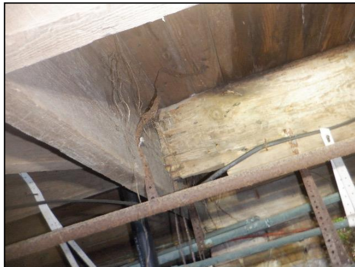
Missing joist hangers
