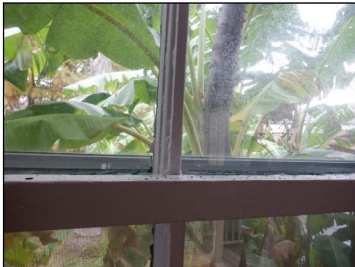
General window issues
