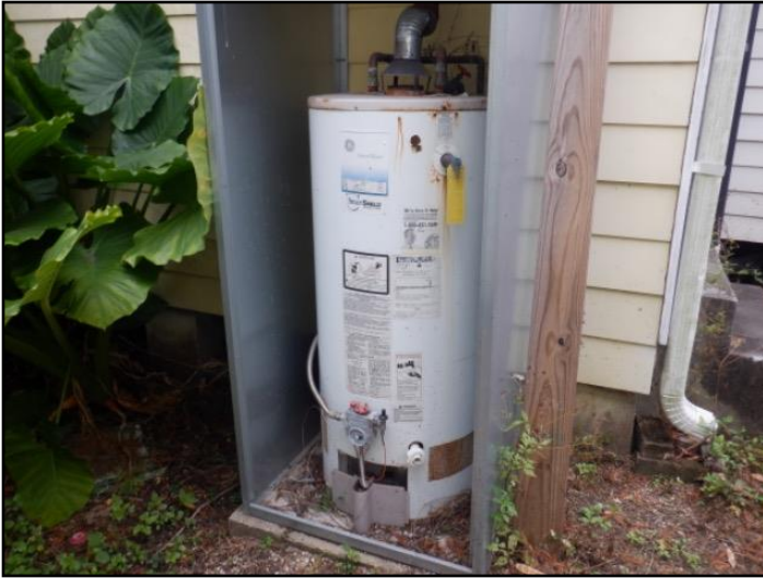
General View of Plumbing System
