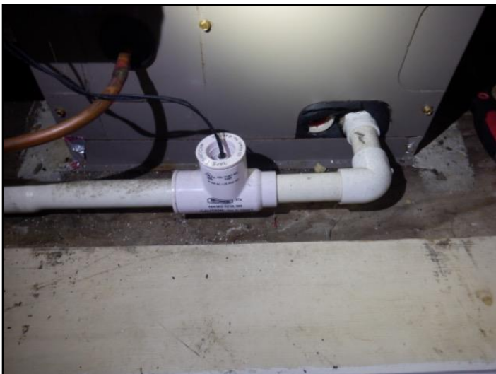
Line not insulated
