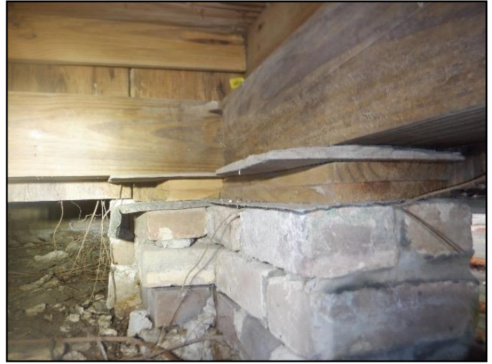
Mortar and/or brick deterioration
