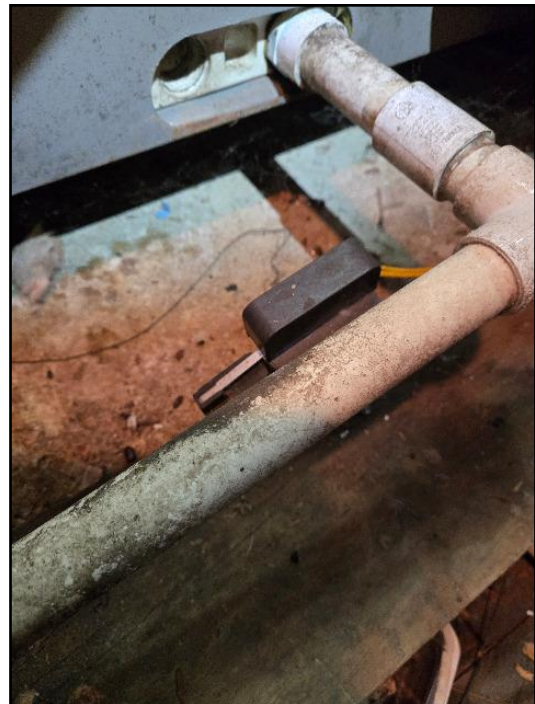
There is a float switch installed on the...
