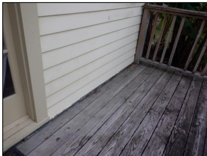
Missing flashing at deck/porch connection
