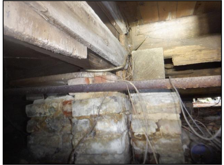
Excessive, or improper shims
