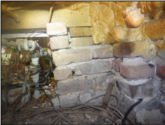
Loose or missing brick or block
