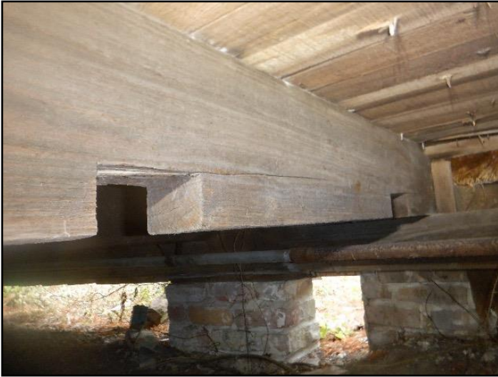
Split or damaged
