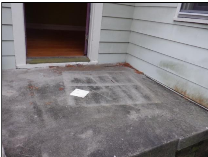
Missing flashing at deck/porch connection
