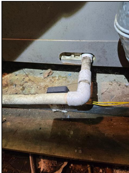
No safety switch
