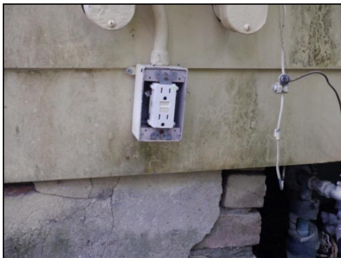
Exterior outlet missing weather cover
