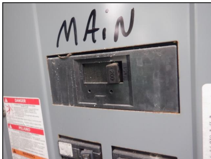
General View of the Electrical System
