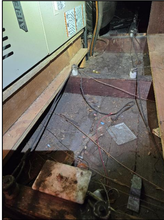
Inactive knob and tube wires found
