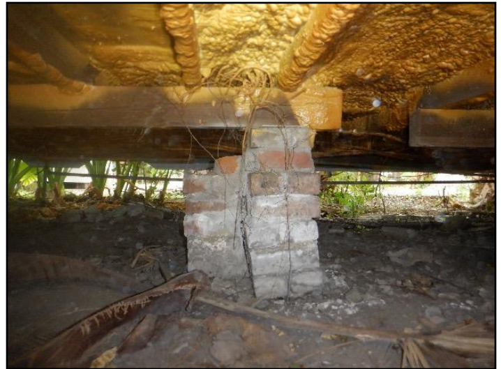
Loose or missing brick or block
