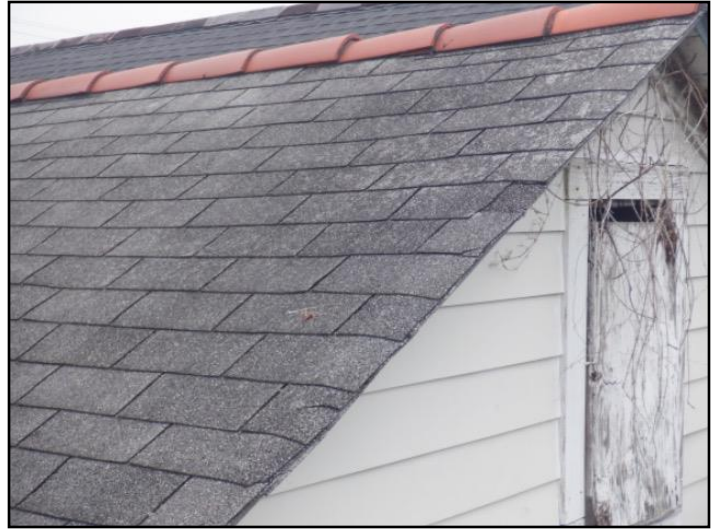
Missing, loose or torn
