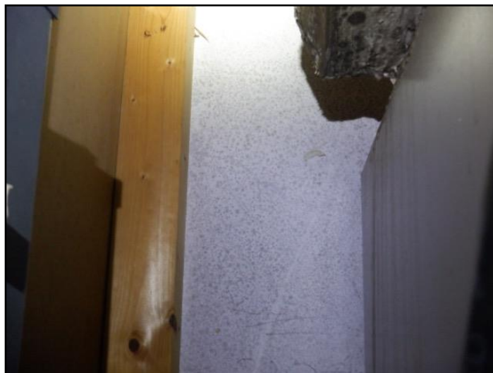
Moisture/mold in closet or air return
