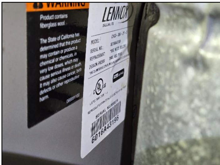
General View of the Cooling System
