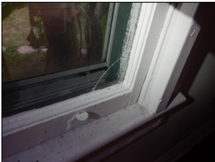
General window issues
