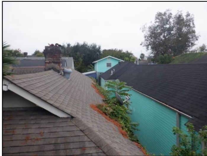
Satellite TV dish attached to the roof...
