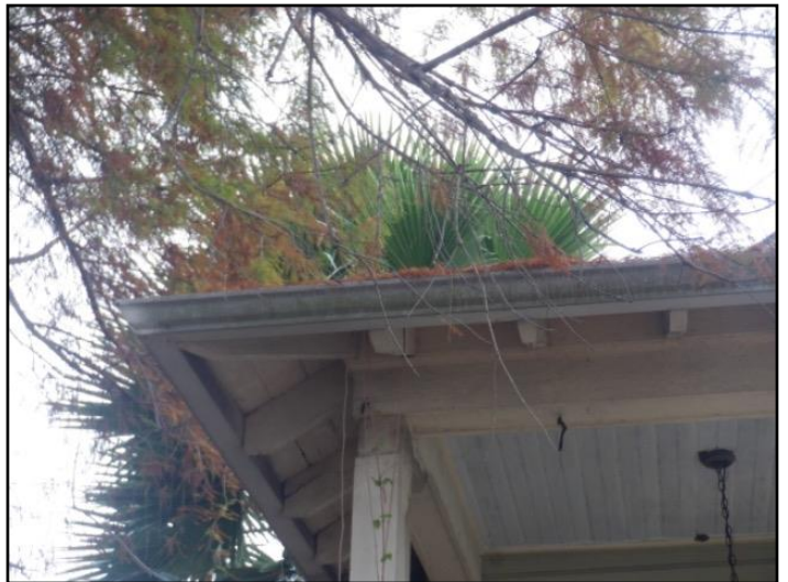
Trees or shrubs too close to building
