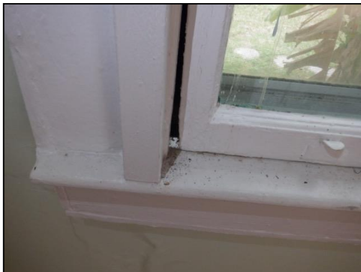
General window issues
