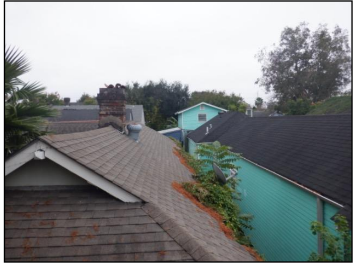
Vines on roof covering
