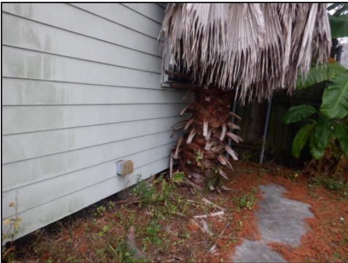
Trees or shrubs too close to building
