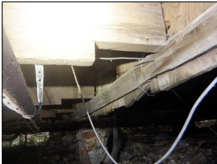
Inadequate end bearing
