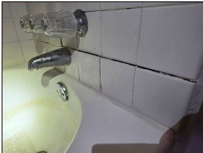
Tile loose, cracked or missing
