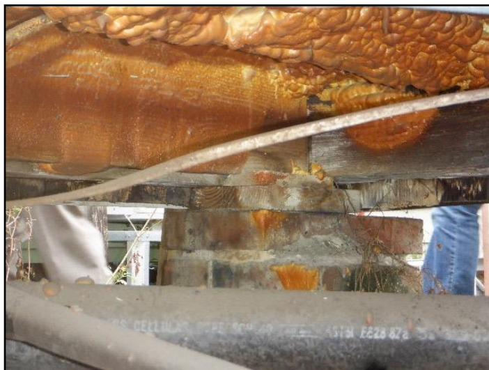
Excessive, or improper shims
