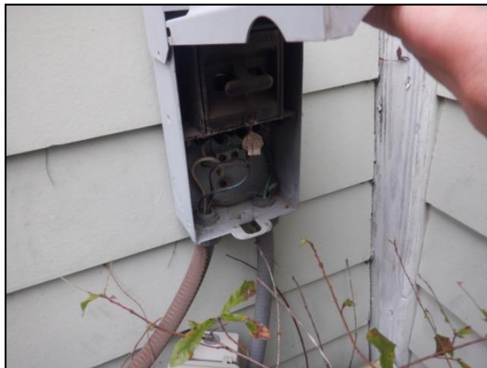
Cover loose or missing
