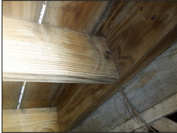
Missing flashing at deck/porch connection
