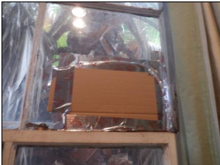
General window issues
