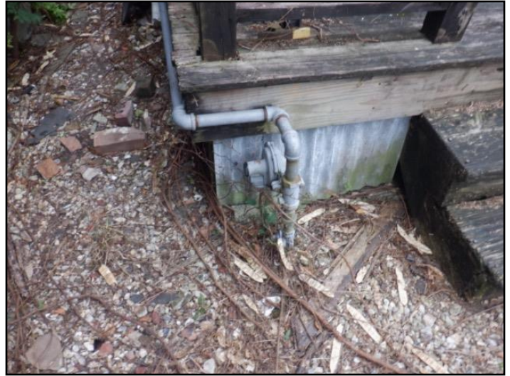
General View of Plumbing System
