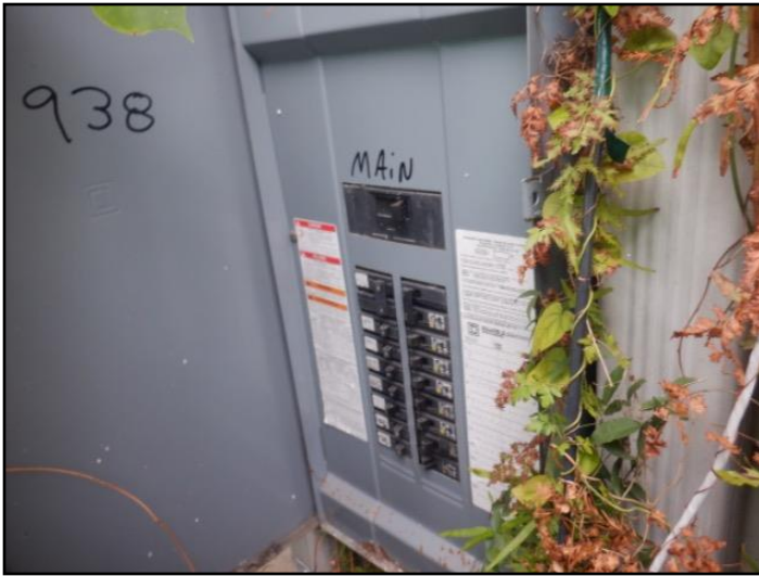
General View of the Electrical System
