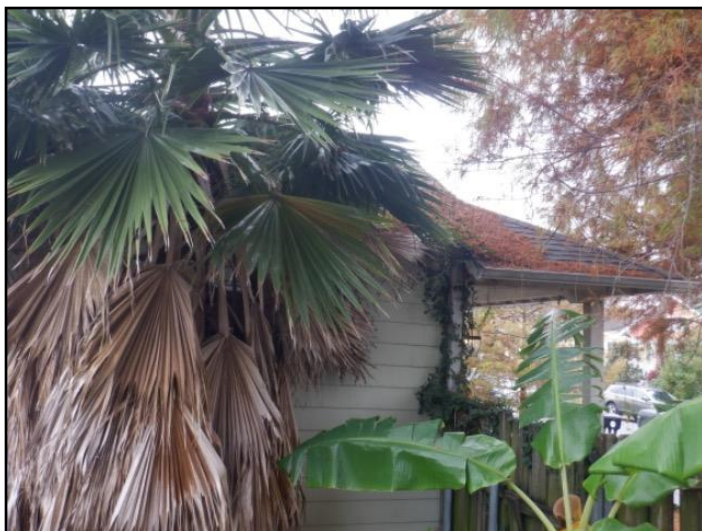
Tree branches touching roof
