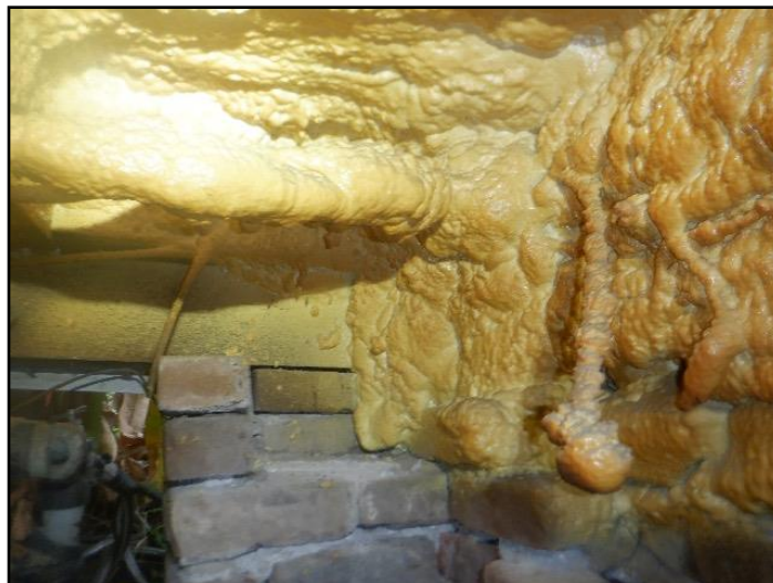
Crawlspace insulation severely limited...
