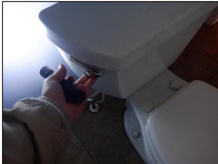
Flush handle loose
