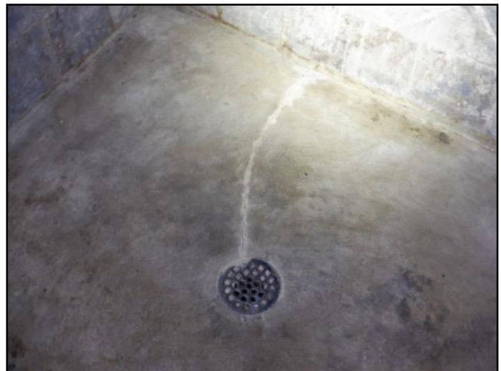
Grout/caulk loose, missing or deteriorated
