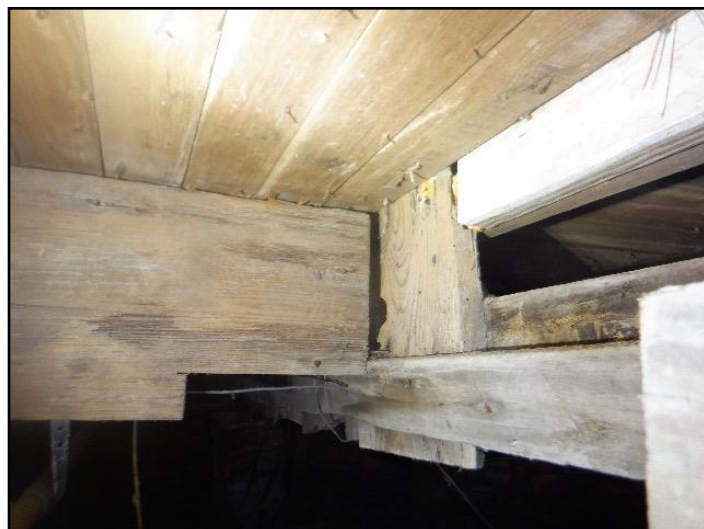
Inadequate end bearing
