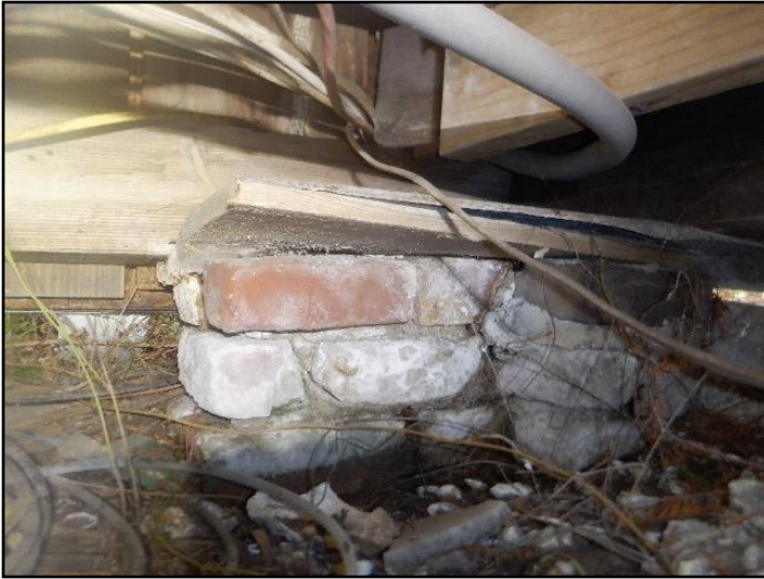
Loose or missing brick or block
