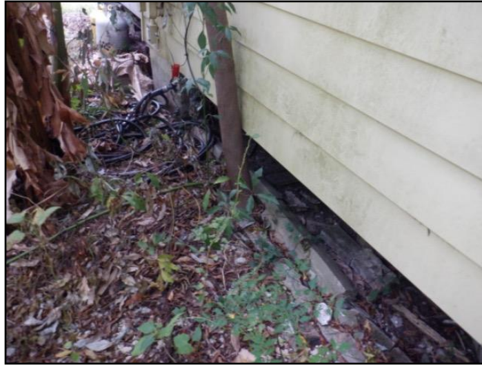
Trees or shrubs too close to building
