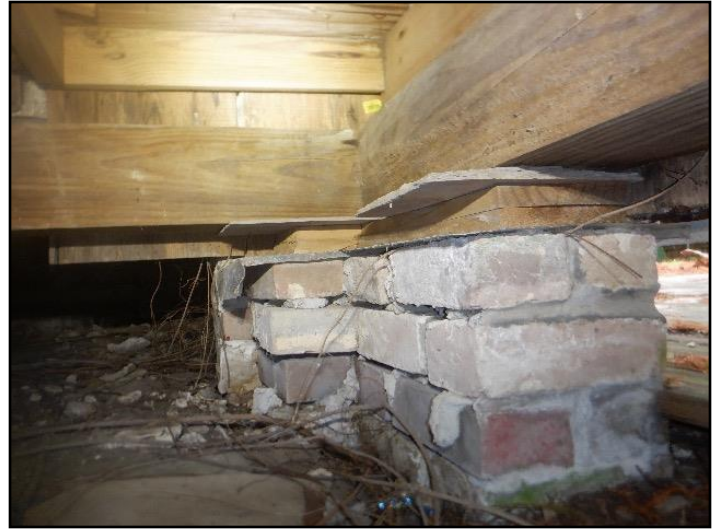
Excessive, or improper shims
