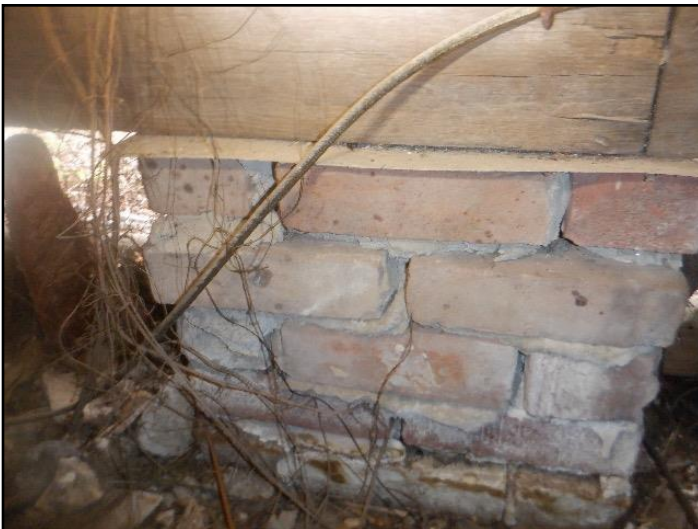
Mortar and/or brick deterioration
