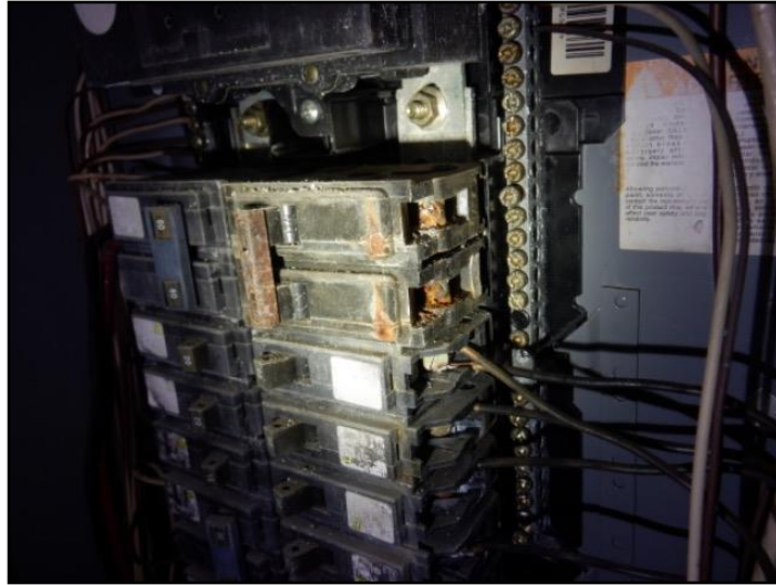
Rust or water in panel
