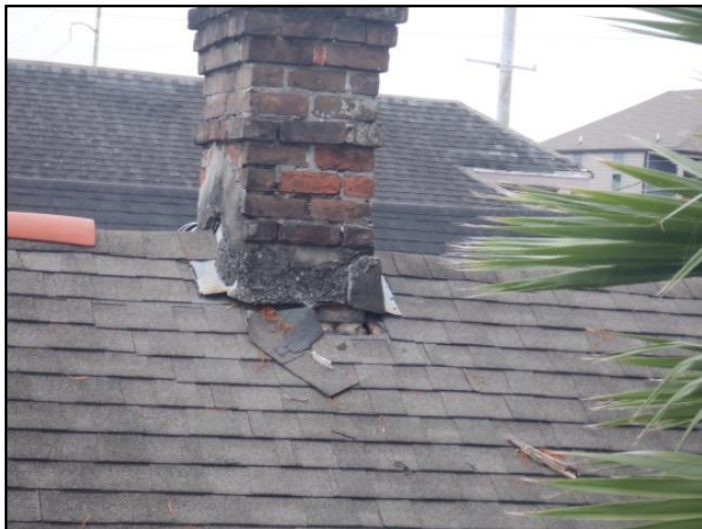
Not let into mortar joints
