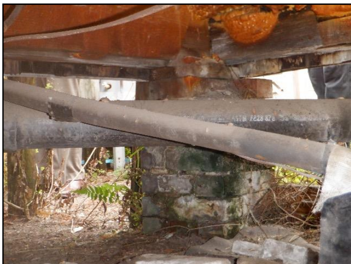
Mortar and/or brick deterioration
