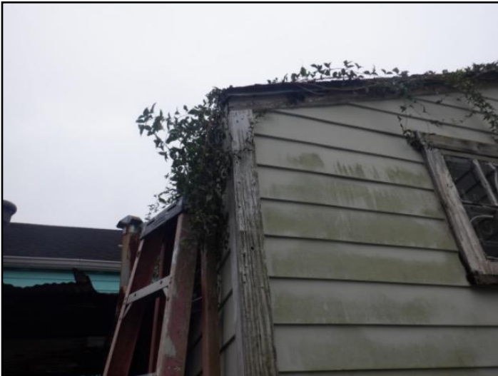
Vines can damage siding by trapping moistur...
