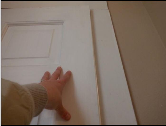
General door issues
