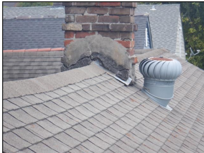
Not let into mortar joints
