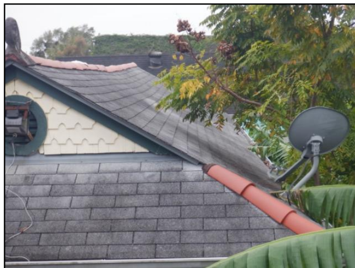
Tree branches touching roof
