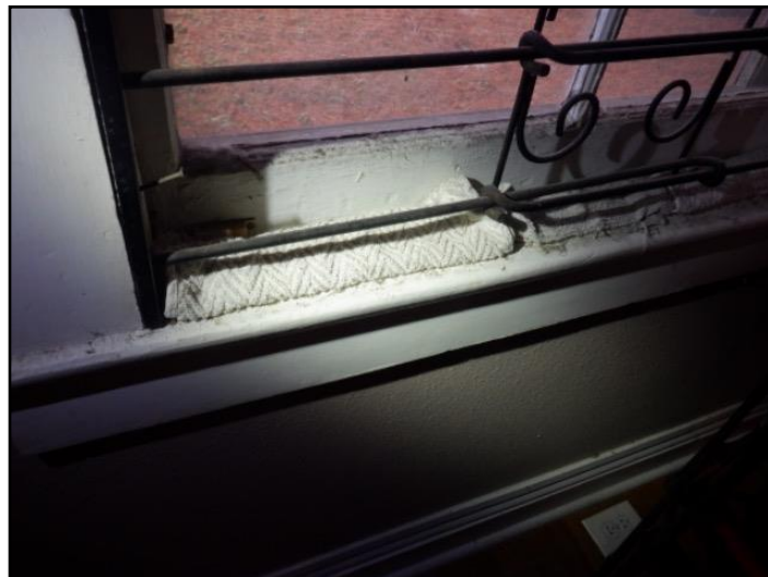
General window issues
