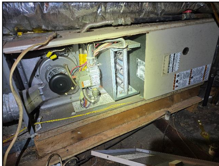
General View of Heating System
