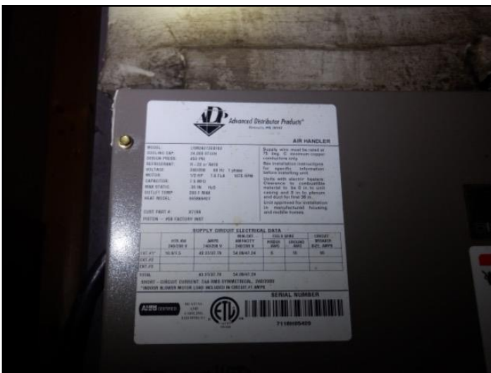
General View of Heating System
