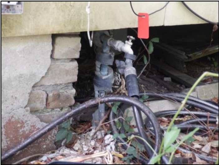
General View of Plumbing System
