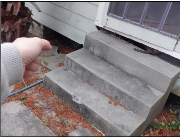
Missing stair handrail
