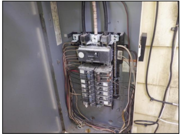
General View of the Electrical System
