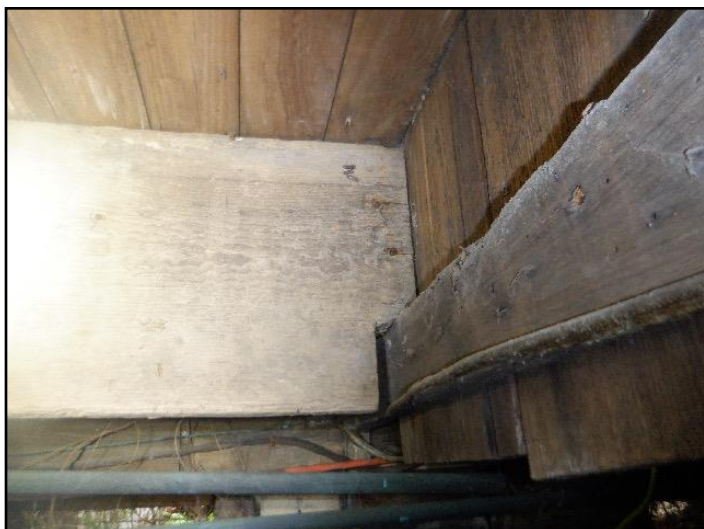
Inadequate end bearing
