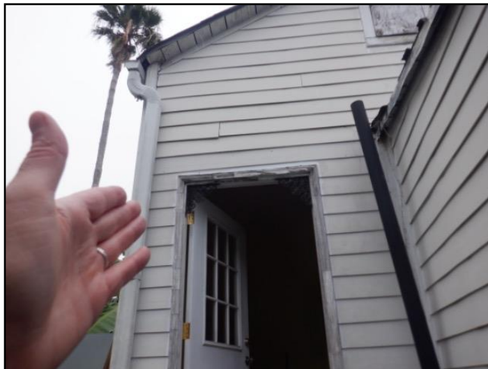
Doors are susceptible to water intrusion...
