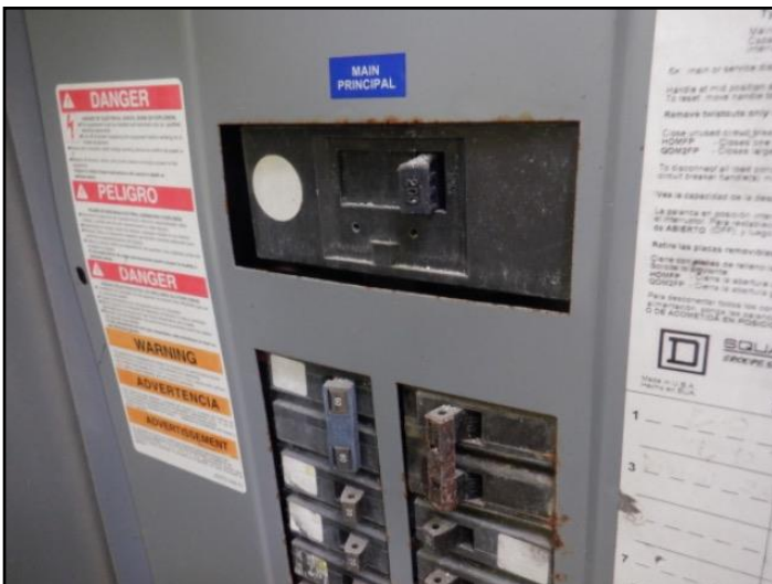
General View of the Electrical System
