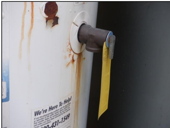
Discharge tube missing
